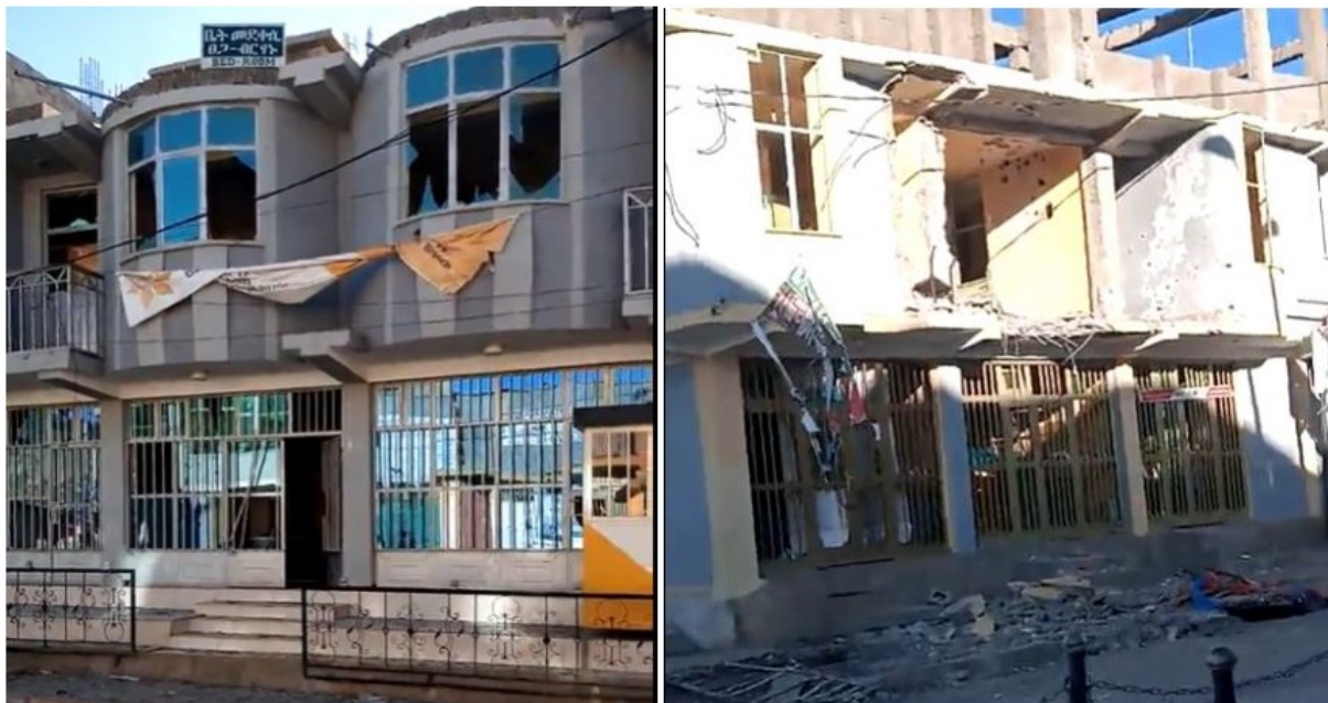
Pictures showing buildings destroyed on the main road of Hageresalam
